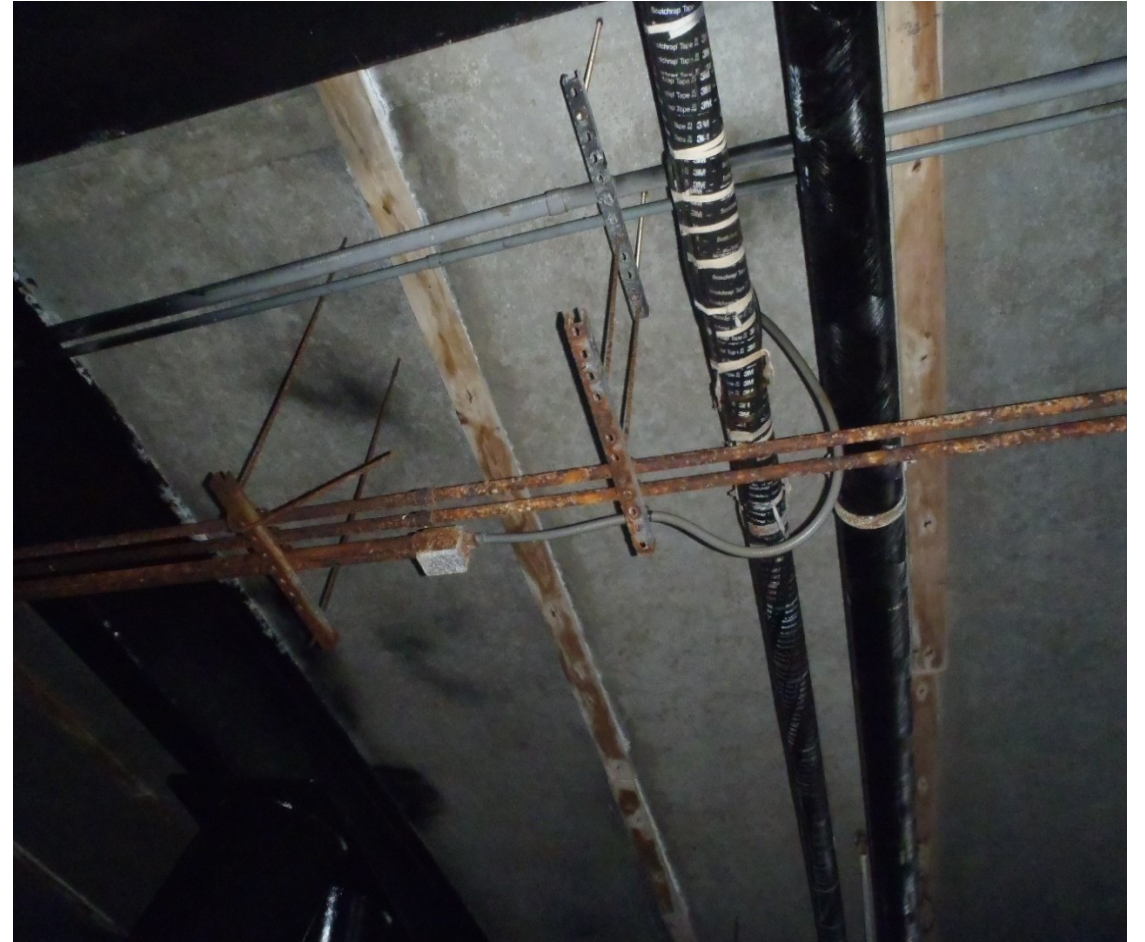
Corroded Electrical Conduits
