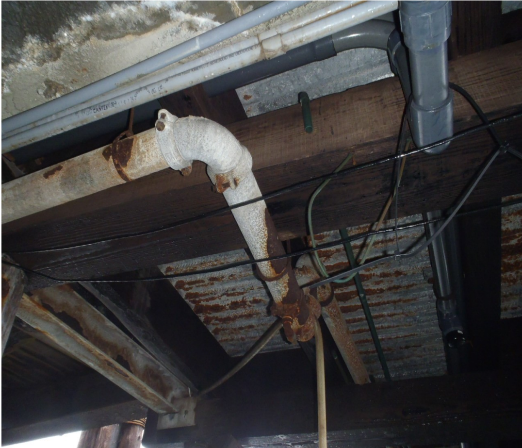
Galvanized Water Main
