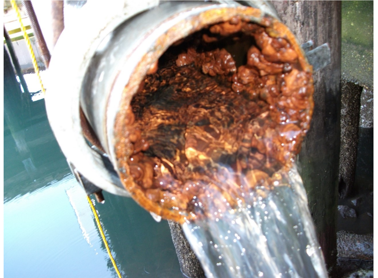
T91 Potable Water Pipe with Similar Age to P69 Pipe
