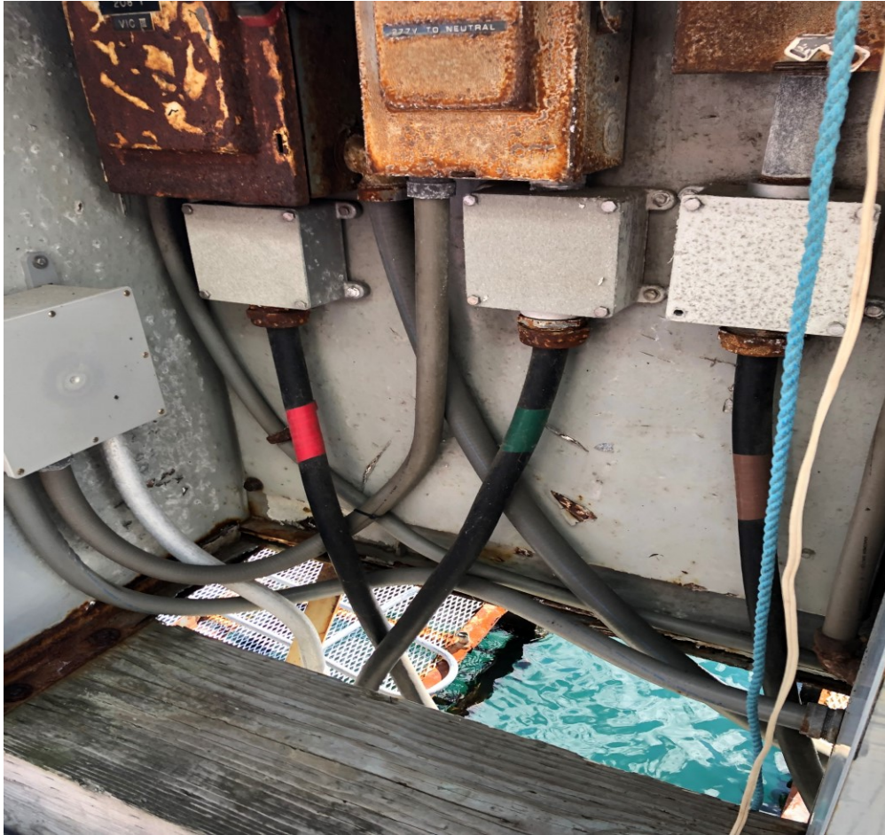
Corroded Electrical Equipment
